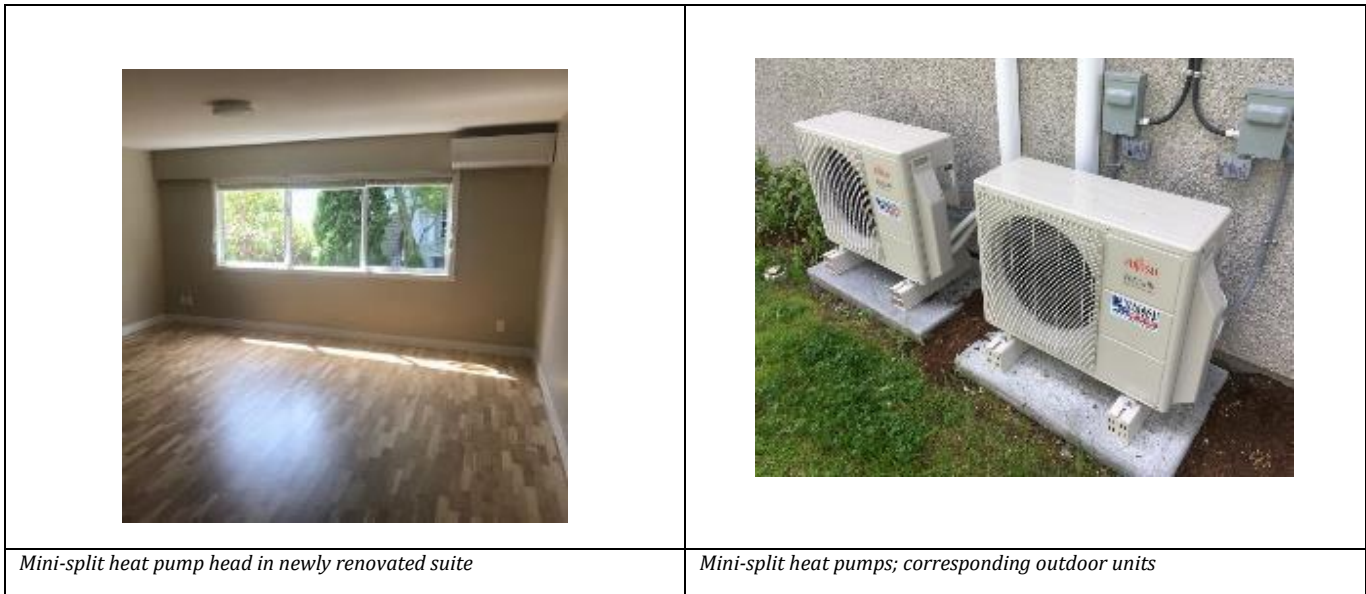
Figure 8: Photos of Mini-split heat pumps replacing a central hydronic system
