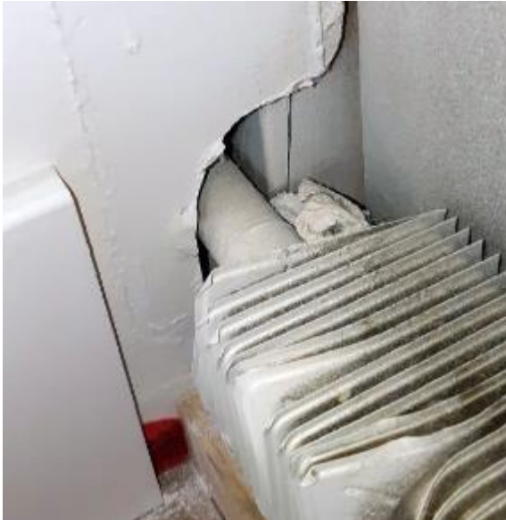
Typical unsealed radiator pipe through drywall
