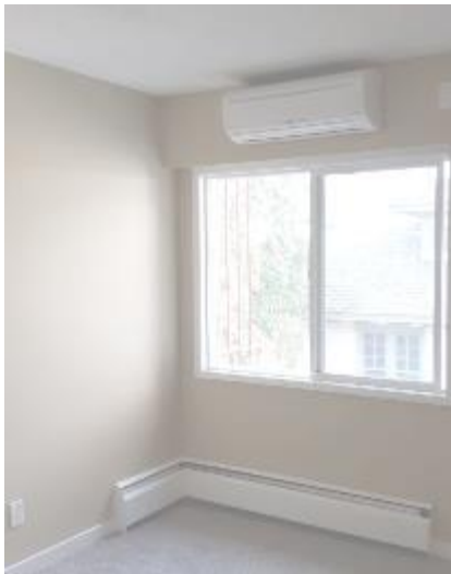
Mini-split head above and hydronic baseboard below
