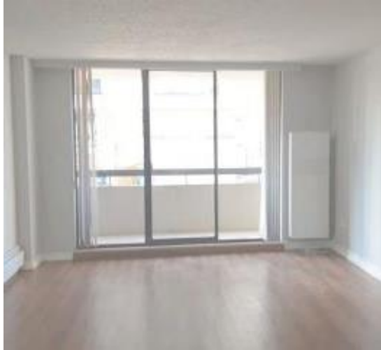
Overview of suite interior - the box on the wall is the ASHP
