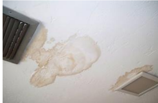
Damage from leaky hydronic systems; damaged ceiling drywall
