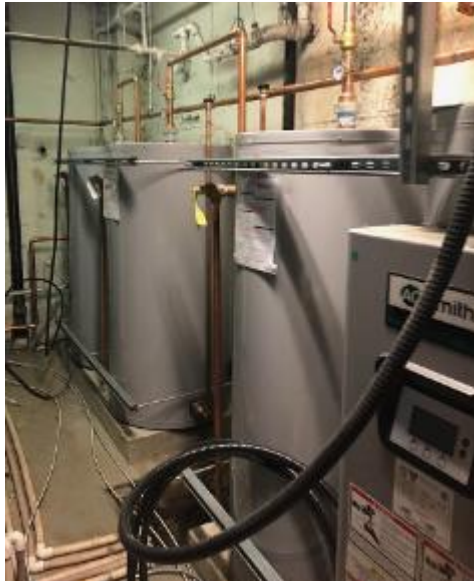
Example of hot water storage tanks and electric resistance backup tank heater
