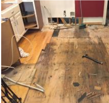
Damage from leaky hydronic systems; damaged flooring
