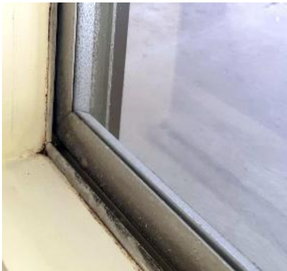
Typical single pane aluminum window; cold and drafty and causes mold and water damage on sills
