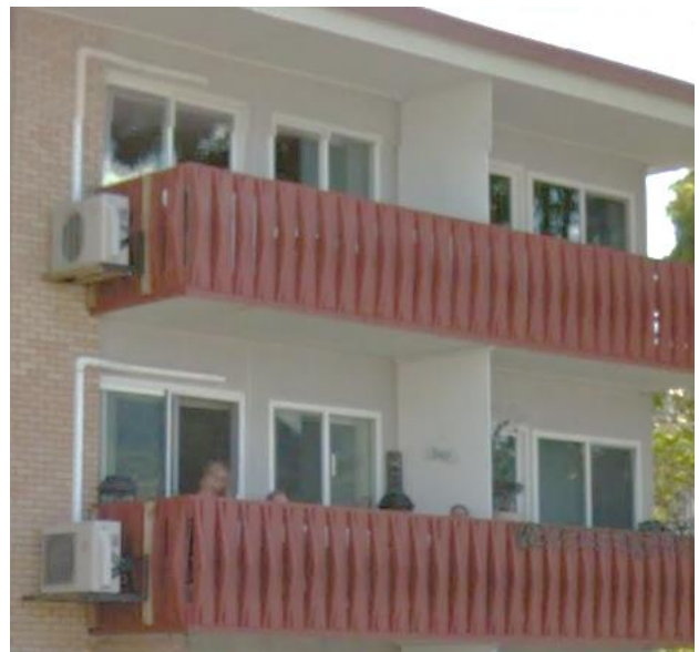
Outdoor unit mounted on the side of the balconies, good solution for low rise buildings (Image credit: Google Maps)
