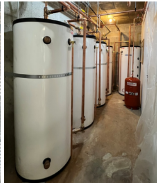
Hot Water Storage Tanks
