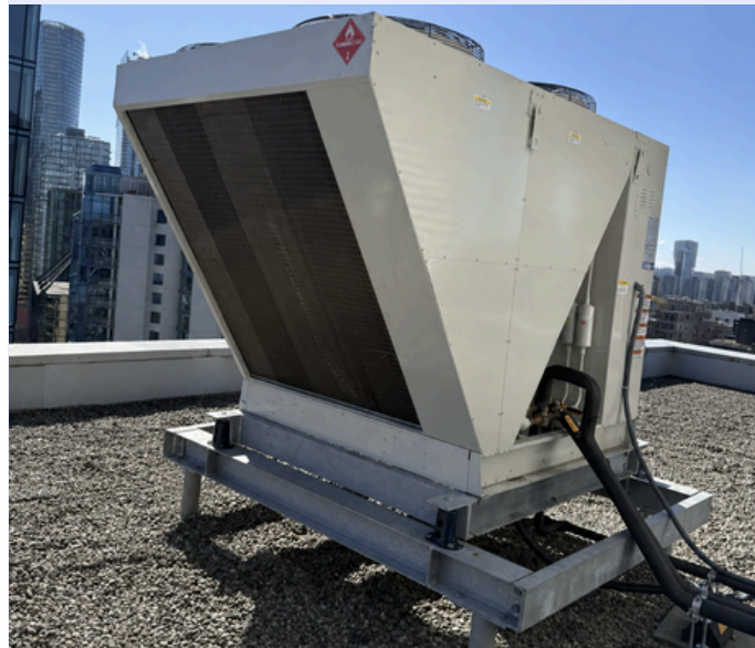
Heat pump make-up air condensing unit
