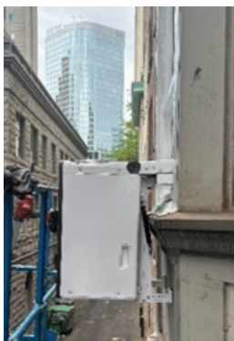
WMHP exterior unit, side view
