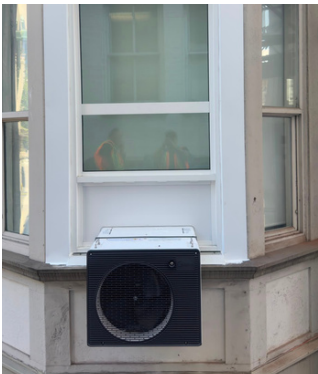
WMHP, exterior unit
